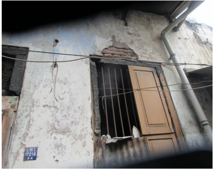
Figure 4. Neglected house due to fire incident (Image by author, 2019)
